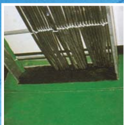
For Cable Tray(slab)
