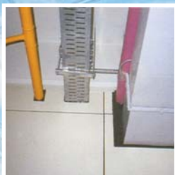
For Pipe and Duct Way
